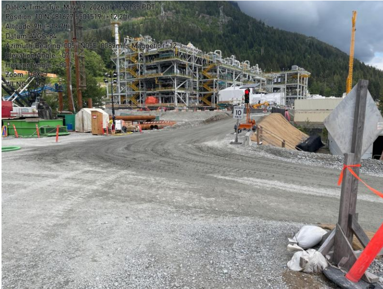
Photo 9. Saturated access road.
