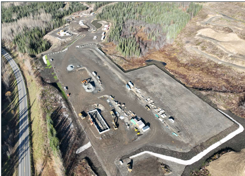
PHOTO 2-34: TREATY SWITCHING STATION WITH HWY 37 ON THE LEFT
