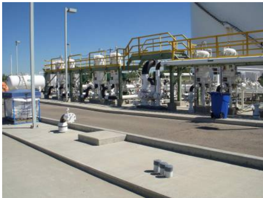
Photo 2.4.8 Typical Fuel Handling and Pump/Filter Areas.
