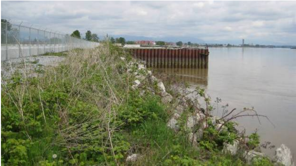
Photo 2.7.3 Marine Terminal Wharf from Downstream on the South Arm of the Fraser River (May 8, 2009)
