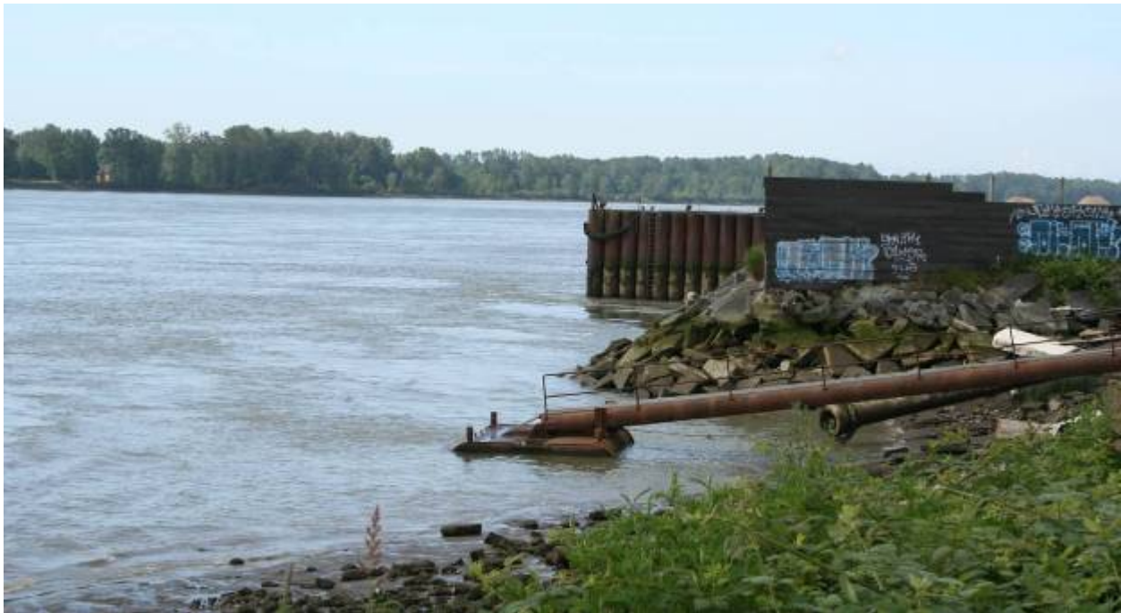
Photo 2.7.1 View of Marine Terminal Wharf and Shoreline on the South Arm of the Fraser River from Upstream (June 22, 2010)
