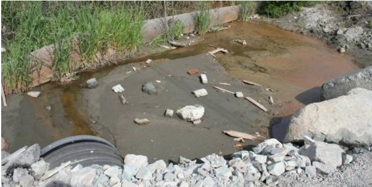
Photo 2.7.5 Standing water in ditch between Triangle Road and entrance to ACME Landfill & Peat Ltd. (the proposed fuel receiving facility site) (June 22, 2010)
